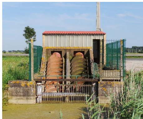
Station de relevage
